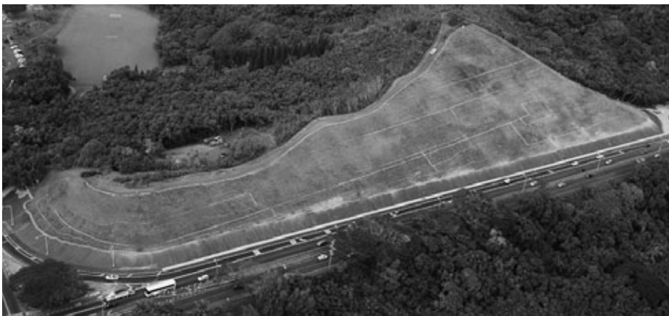
Kalaniana'ole Highway Emergency Landslide Repairs Project at Castle Junction by Parsons, Brinckerhoff Queade & Douglas, Inc.
