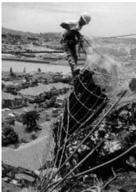
Earth Tech: Laea Emergency Rockfall Remediation project. Demolition under mesh to remove large, loose boulder.
