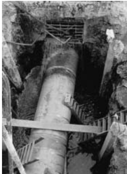
Belt Collins: Waipahu Wastewater Pump Station project. Application of unique construction techniques prevented contamination of groundwater.
