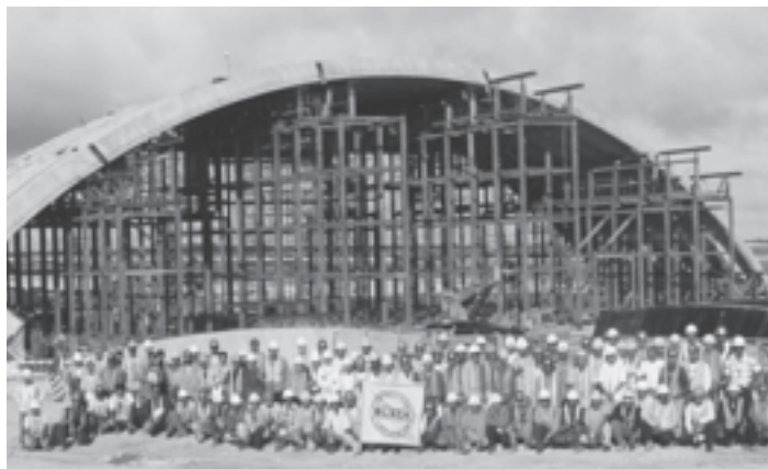
OCEA Award Winning Project: Design-Build AEF FOL Aircraft Maintenance Hangar, Andersen Air Force Base, Guam.
