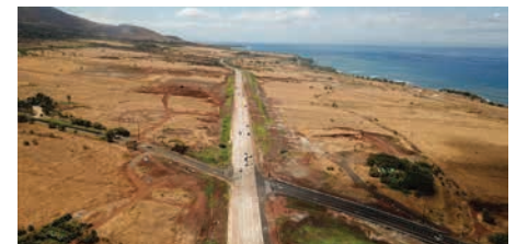
Honor Award, Completed Lahaina Bypass Phase 1B-2 at Hokiokio Place intersection (facing south).
