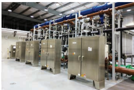
Excellence Award, Membrane Filtration Units with Control Panels in the Completed Iao WTP
