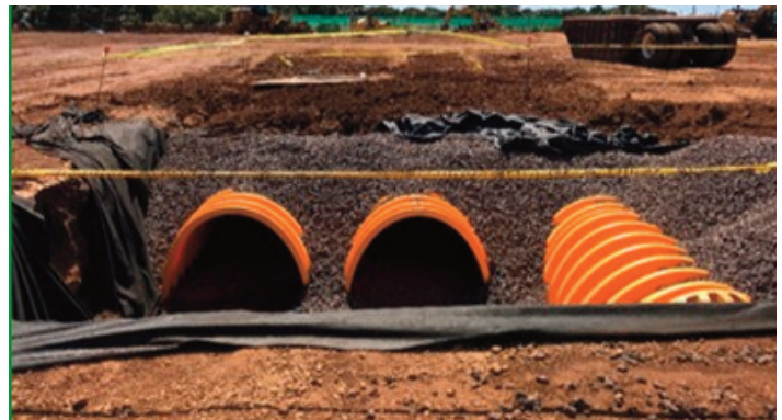
Honor Award: Installation of underground detention basin intended to capture excess storm water runoff generated by the site.
